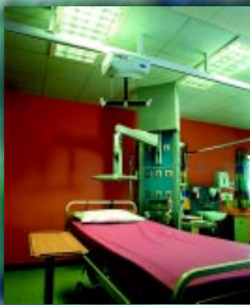
A ceiling track hoist ensures patient and carer safety
